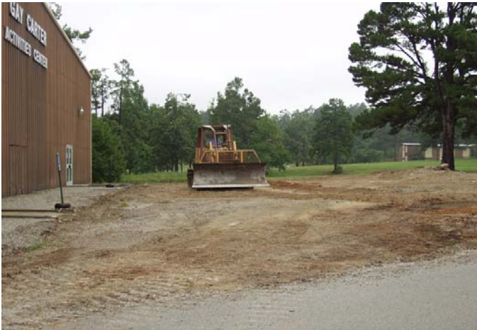
Student Center construction begins as front addition to Gay Carter Activities Center.
